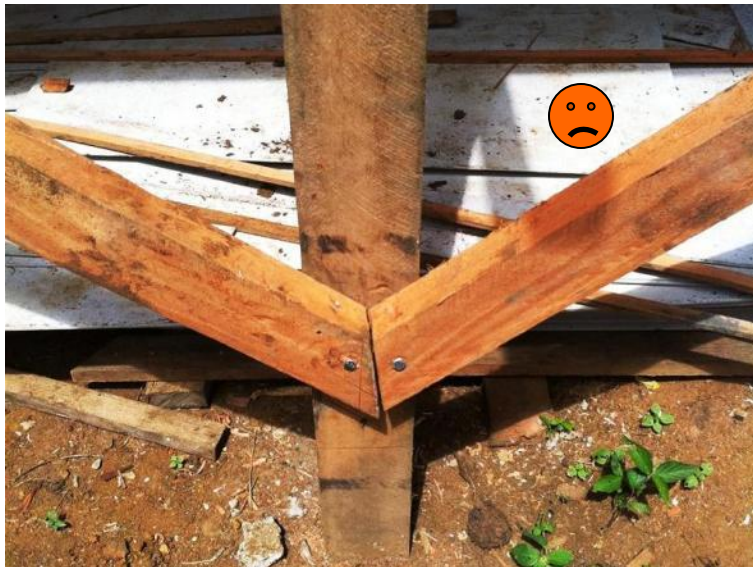
Bolts too close to the end of timber brace Papua New Guinea (Mt Hagen)
