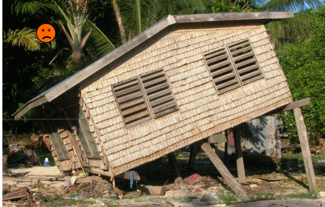
Inadequate Bracing (Solomon Islands)
