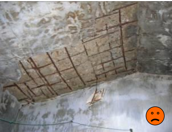
Suspended concrete roof corrosion (India)
