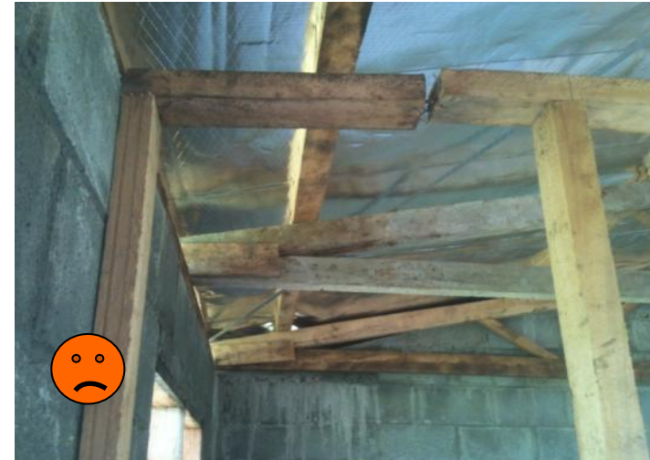
Inappropriate Joint in Top Plate – PNG
