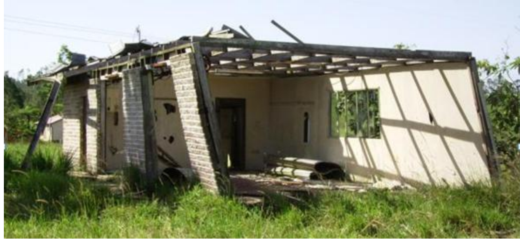
Photo: Cyclone Damage on Aitutaki in the Cook Islands Courtesy of D Kaunitz (Emergency Architects Australia)
