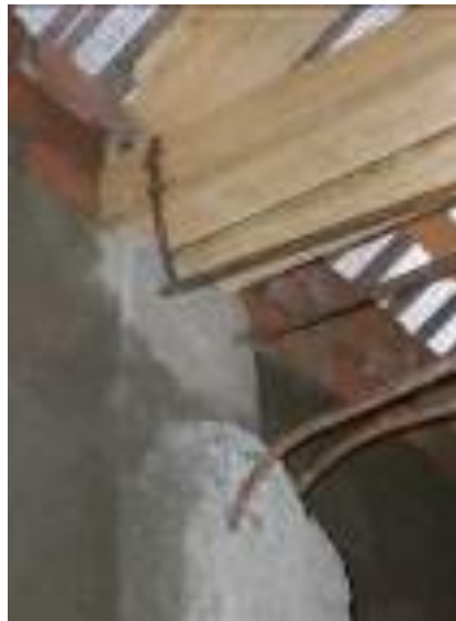
Bent reinforcement – Aceh
