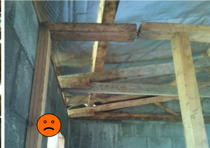
Inappropriate Joint in Top Plate – PNG
