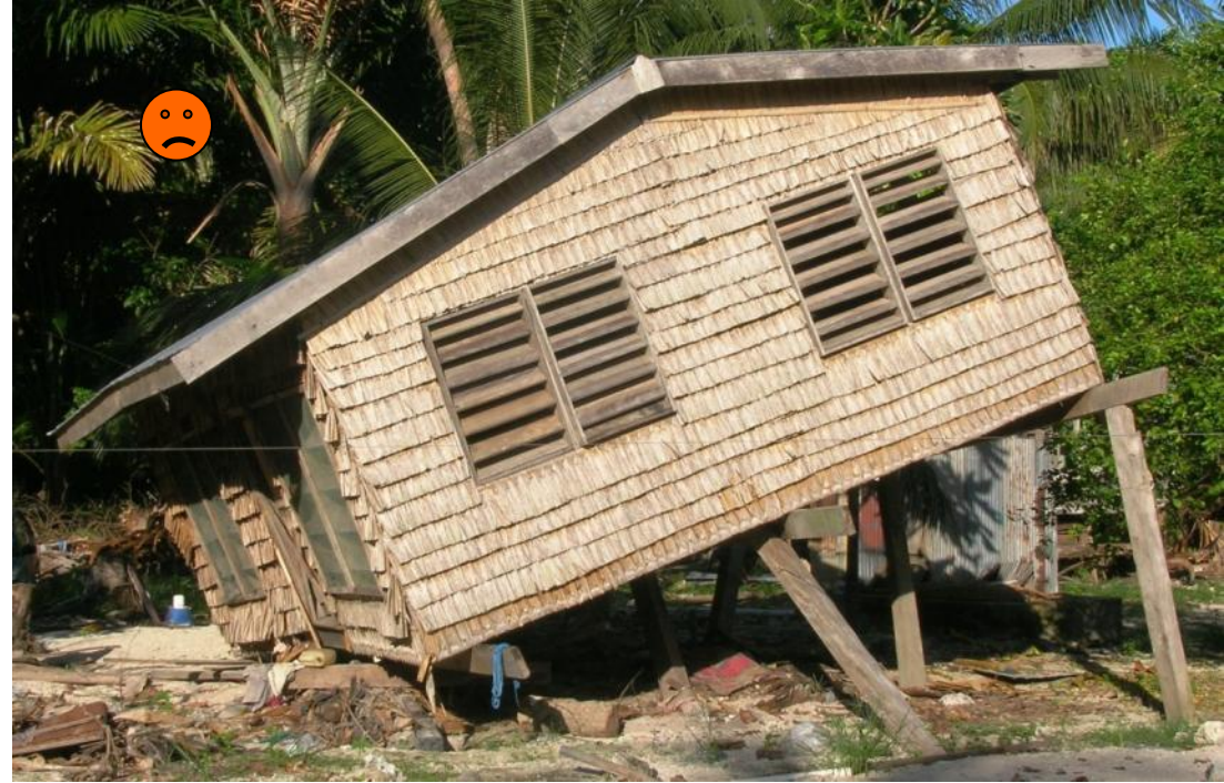
Inadequate Bracing (Solomon Islands)
