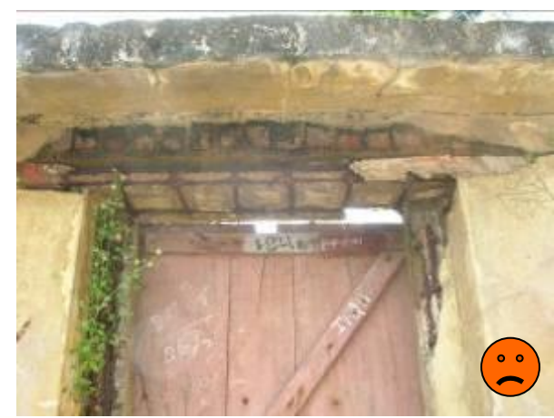
Concrete lintel reinforcement corrosion (India)
