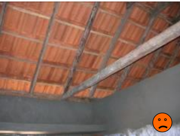
Tiles not tied down – India
