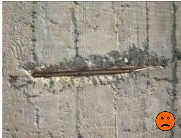
Concrete wall corrosion (Australia)
